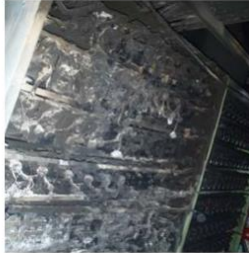
Figure 2 – Battery cabinet with doors removed. Damage within left cabinet.
