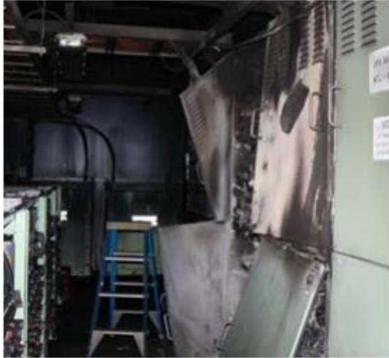
Figure 1 – First entry into the battery room post incident.
