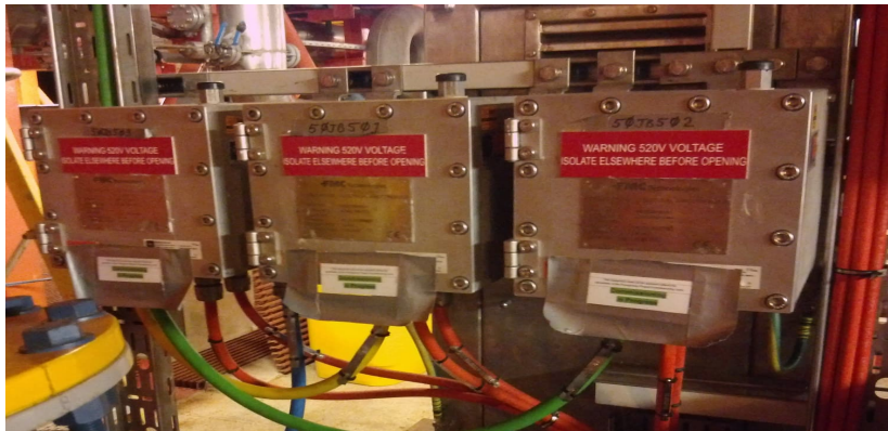
Umbilical Electrical Cable Junction Box
