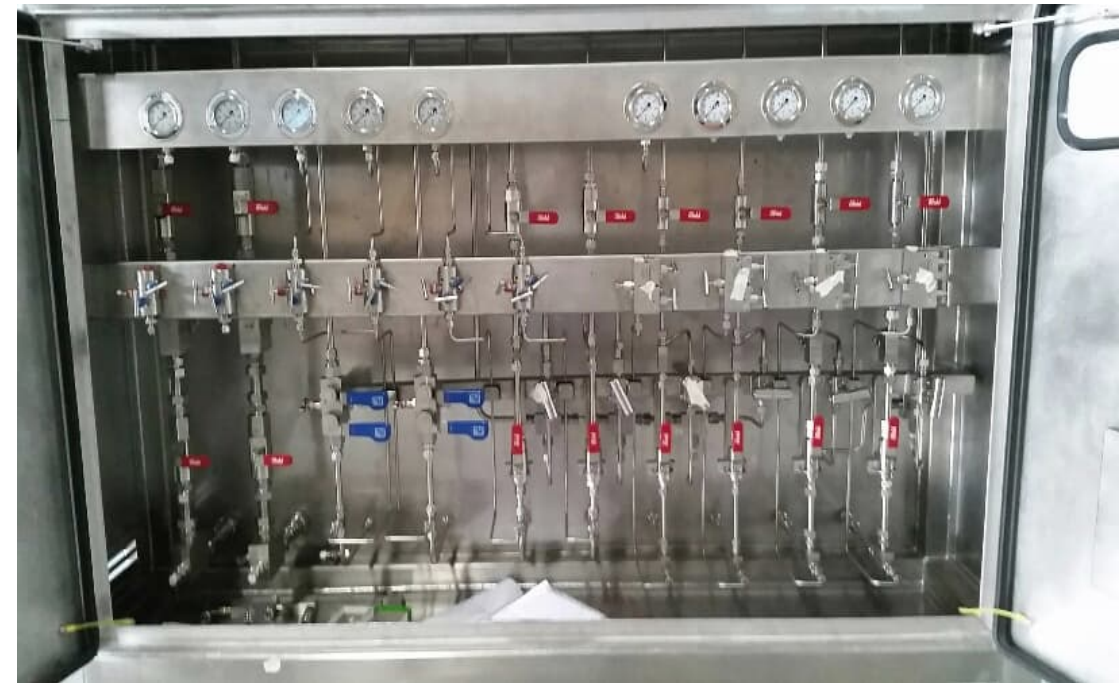
Umbilical Tube Termination Unit
