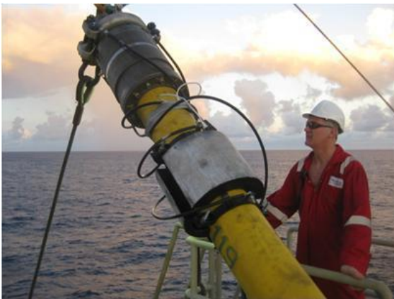
Figure 56 – Anodes fitted to pipe and connected to EF
